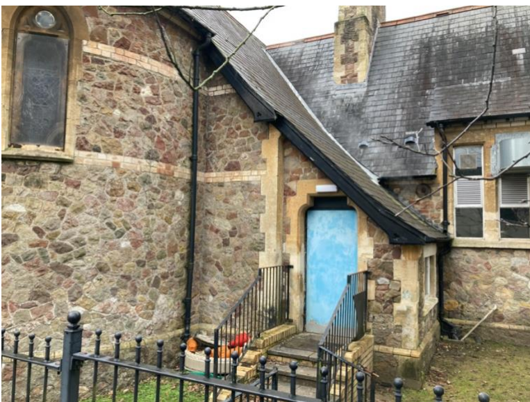
The blue fire door is far from attractive sight from the main road and should be replaced/enhanced.
